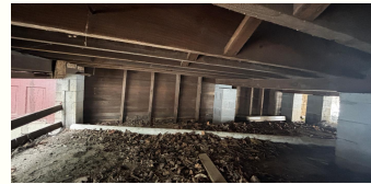
Crawlspace under the south stage wall: leaves on bare earth, no vapor barrier.
