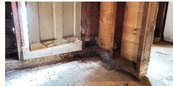
Rotted sills, east entrance interior — daylight where structure used to be.
