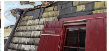
West window at foundation level; moss has colonized the lower cedar shingles.
