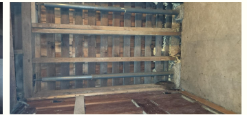
Interior west corner — two blue steel jacks are currently holding load.
