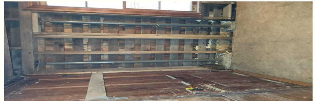
Interior west foundation corner. The two blue posts are temporary steel jack shores currently holding load.
