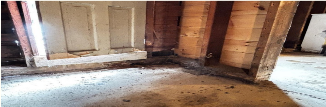
Rotted wood sills at the east entrance, interior. The white box is daylight where structure used to be.
