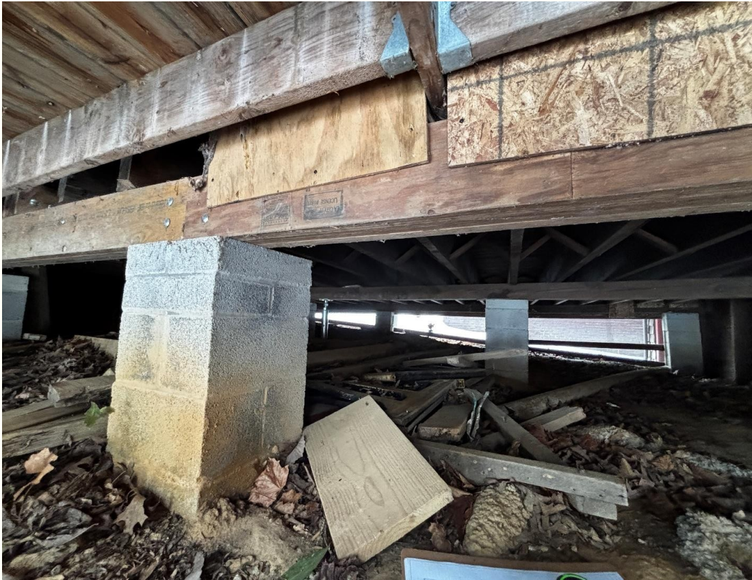
Crawlspace pier — patched. A 19th-century brick pier reinforced with concrete block. The kind of fix that has gotten the Assembly Rooms this far, but isn't the long-term answer.
