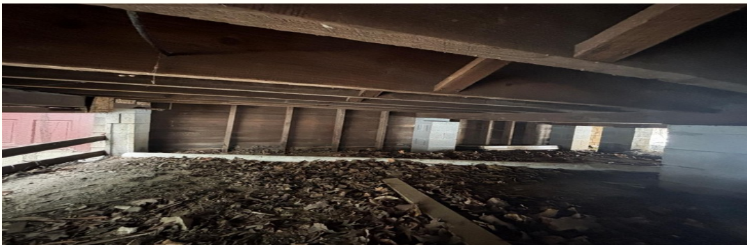
Crawlspace under the south stage wall, looking north. Leaves and bare earth, no vapor barrier.
