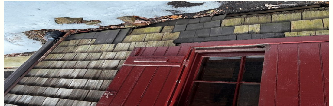
Exterior west window at foundation level. Moss has colonized the lower three courses of cedar shingle.
